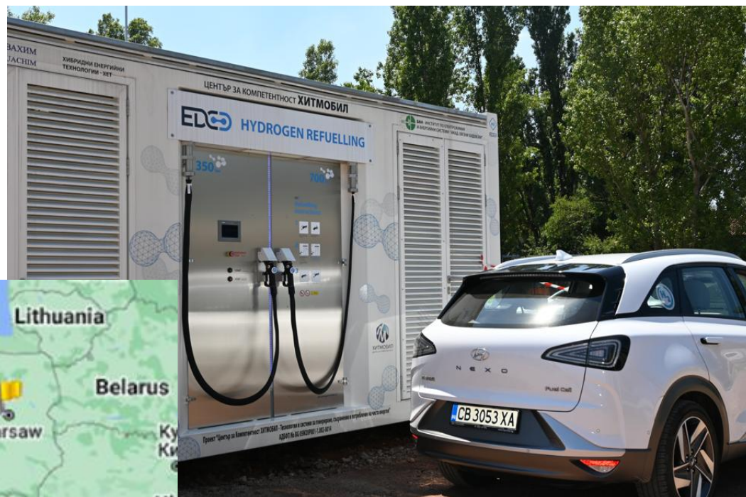
Hydrogen refueling station
